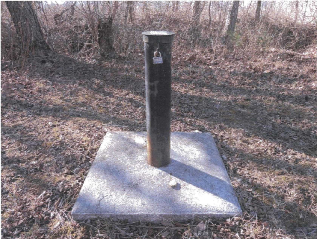
FV groundwater monitoring well MW-202, secured with a lock, clearly labeled and in good condition.
