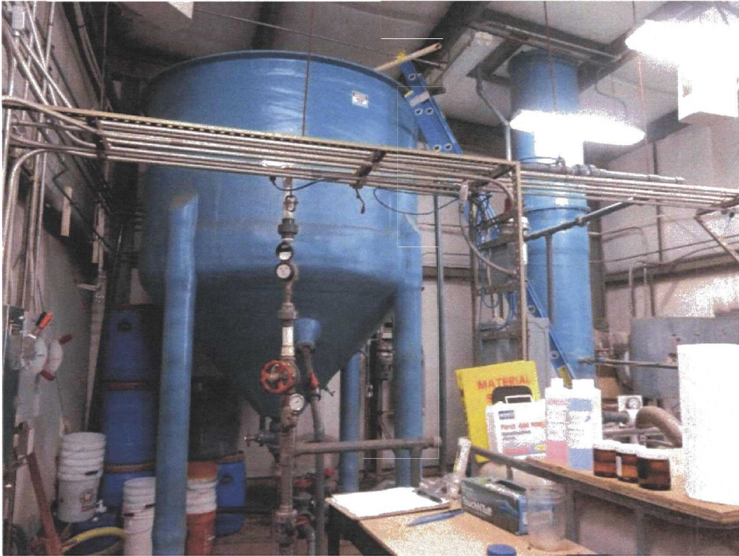
Groundwater treatment system components inside the FV groundwater treatment system building.
