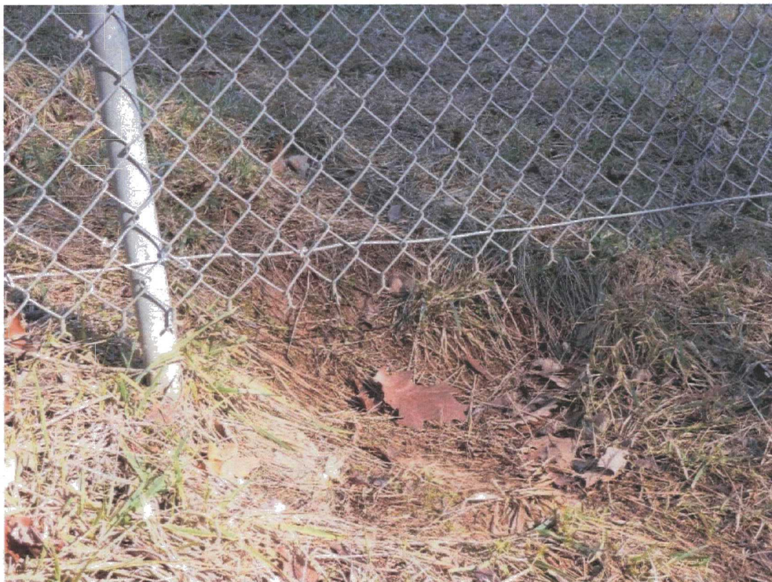
Small dug-out area under the fence that surrounds DA-10-11. Animals sometimes dig under the fence, but do not dig on the surface of the cap.
